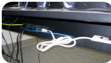
Figure 2 Power strips must not be “piggybacked”. Power strips and electrical devices must be plugged into receptacles. Extension cords can’t be used to provide permanent power.
