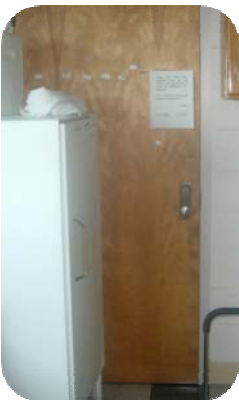
Figure 1 Doors must not be blocked. In the event of a fire room occupants must be able to exit the room quickly.
